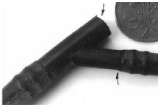
Figure 2: Pipe fracture (upper arrow) from which fuel leaked
